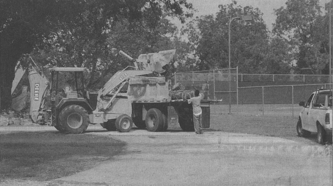
A city crew worked on Tuesday to remove a large tree that fell over at the golf course as a result of the very wet conditions from last week.
